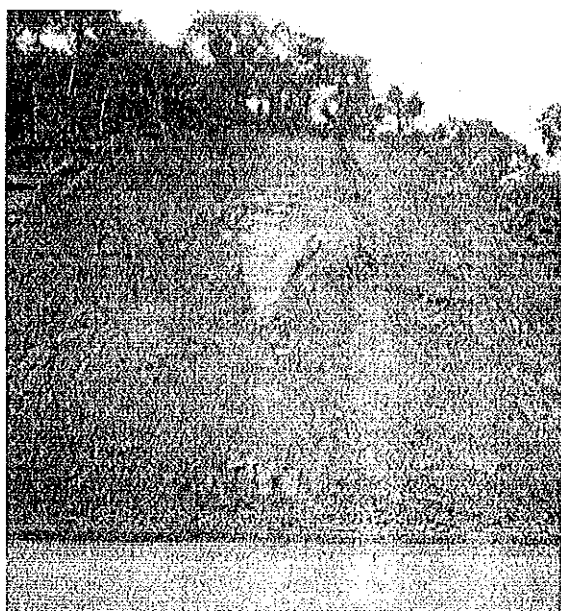
b) Complex slip surface
